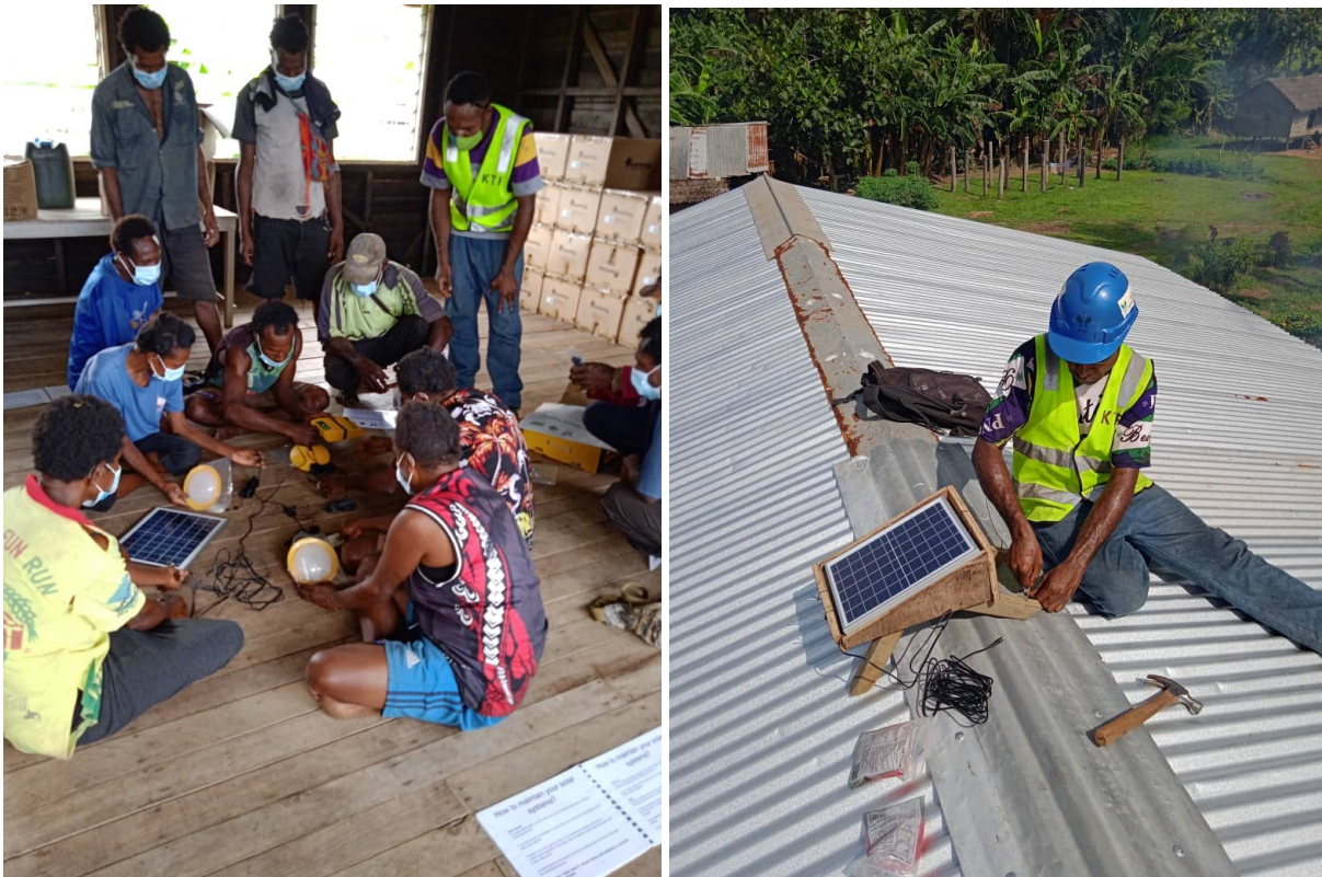
Image 2 and 3: Solar champions being trained by the KTF solar installation team (L) Solar equipment being installed (R)
